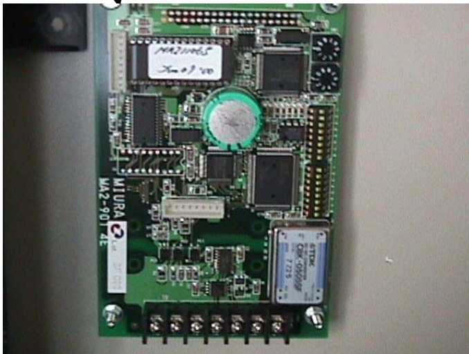
Boiler MA2 Board
